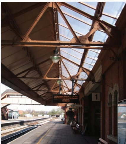
Stratford station recently refurbished with Multi-Link-Panels NF fitted with aluminium sandwich panels on the left and 25mm multiwall polycarbonate glazing on the right
