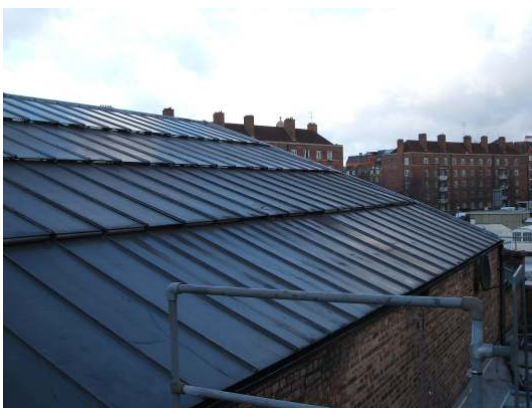
Edgware Station - before with traditional glass
